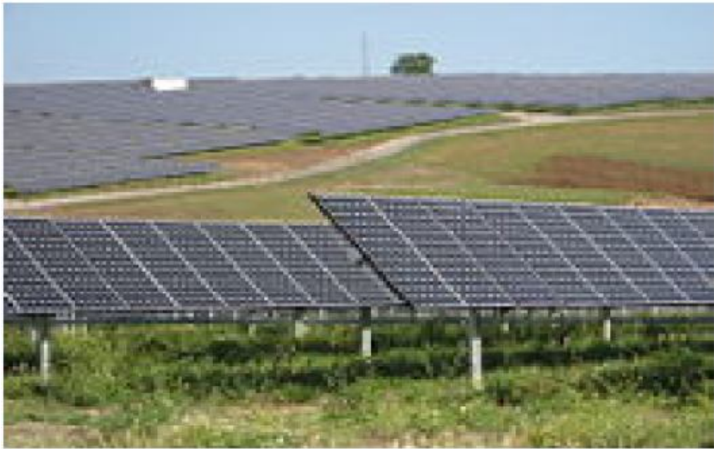
Figure 3: Solar cells power plant. (Ibidapo-Obe and Ajibola 2011)
