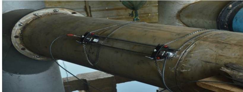
Fig.3 Ultrasonic flow meter mounted on the delivery pipe of vertical submersible pump
