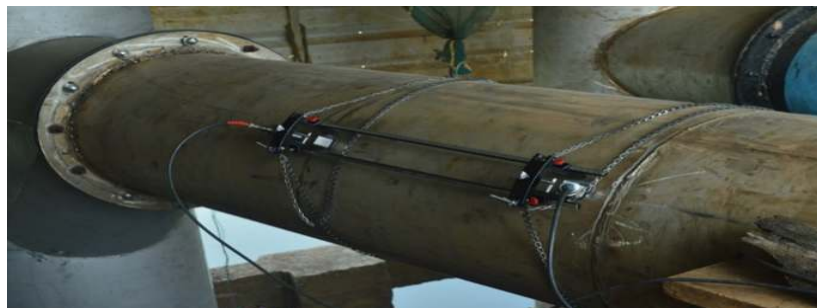
Fig.3 Ultrasonic flow meter mounted on the delivery pipe of vertical submersible pump
