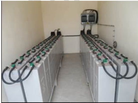
Figure 3: the two battery chains
