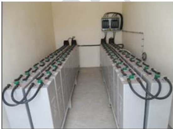
Figure 3: the two battery chains
