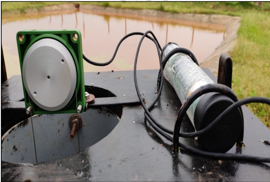
Plate 1b: Close view of thalimed data encoder and data logger used in the study area
