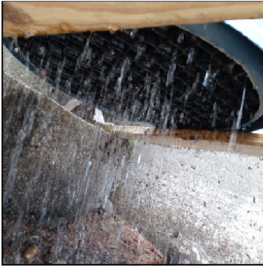
Fig. 4. Bio-tower CF-1900 water Distribution [27]
