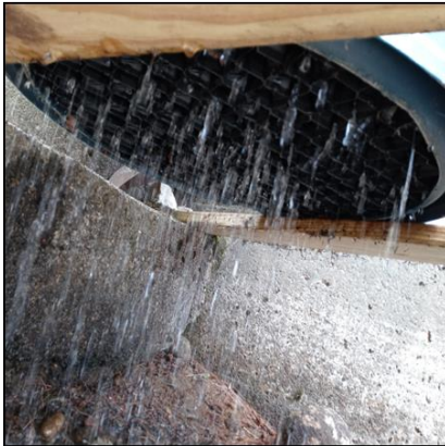
Fig. 4. Bio-tower CF-1900 water Distribution [26]
