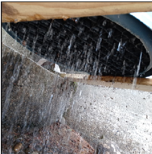
Fig. 4. Bio-tower CF-1900 water Distribution [26]
