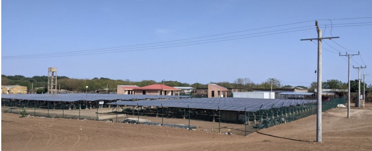
Figure 4.2. A view of the PV MG infrastructure in Omorate, Dasanech district, Southern Ethiopia
