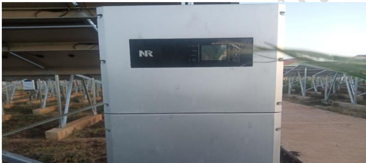
Figure 9. NR-grid tide inverter rating 33kw
