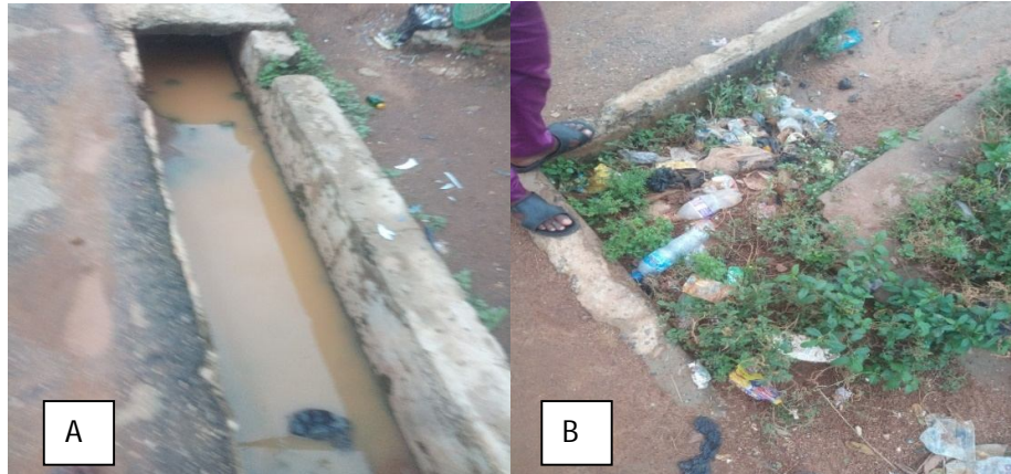
Figure 9A: Water logged drainage at Araromi, B: Blocked Drainage at Owode
