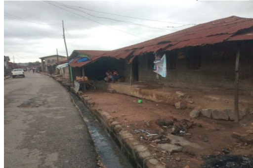
Figure 8: Dilapidated Corrugated Iron Sheet for Building Construction at Araromi
