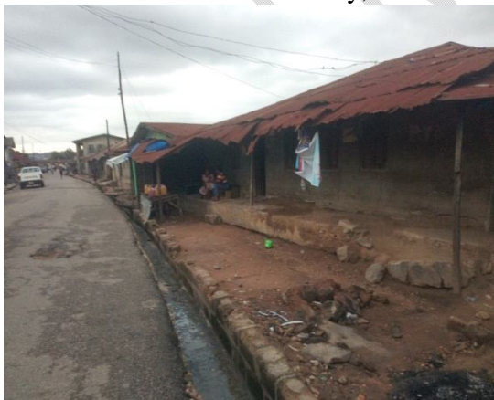
Figure 11: Dilapidated Corrugated Iron Sheet for Building Construction at Araromi
