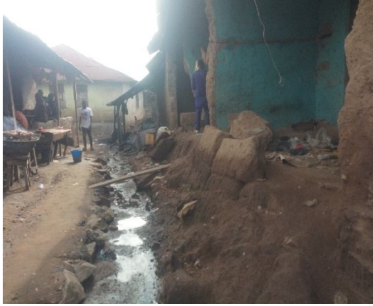
Figure 10: Dilapidated Building Constructed with Mud at Odojoka
