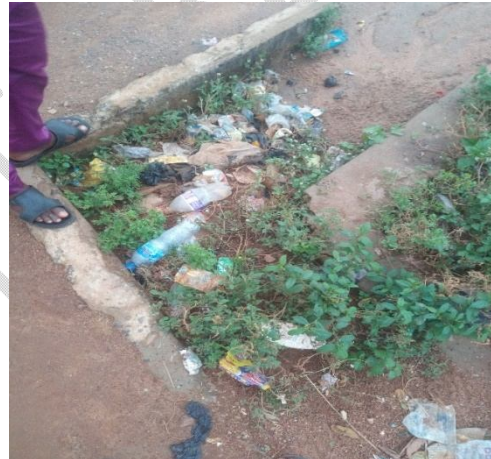
Figure 13: Blocked Drainage at Araromi Owode
