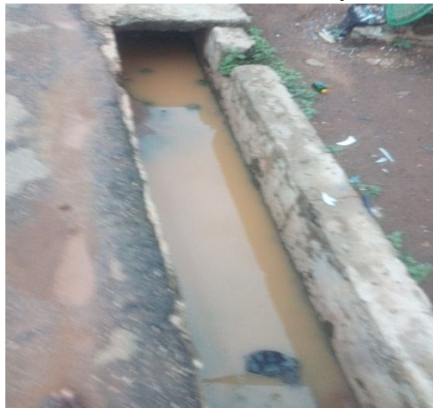
Figure 12: Water logged drainage at Araromi Owode
