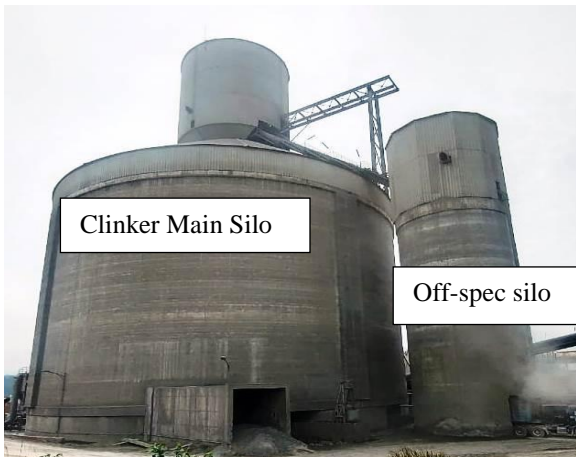
Figure 3: An image of a Main clinker silo and Off – Spec silo in an existing cement plant
