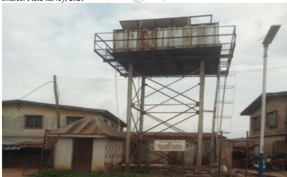
Figure 4: Borehole infrastructure in Iju
