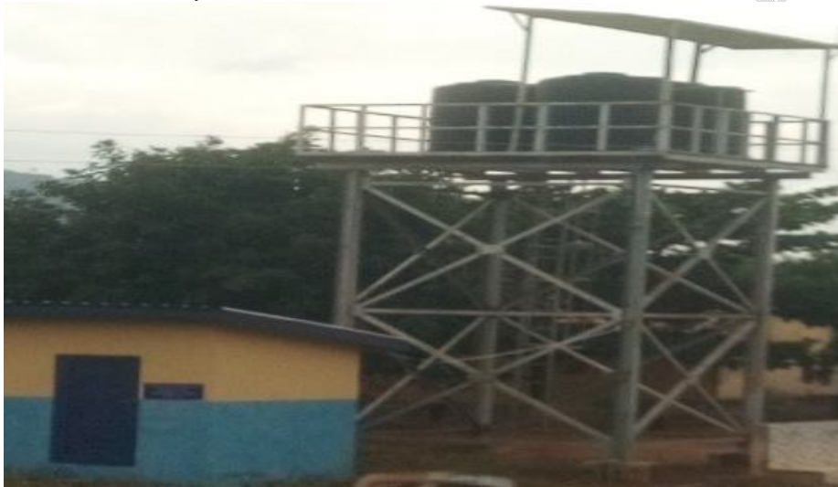
Figure 7: Solar powered borehole in Itaogbolu Source: Field survey, 2021
