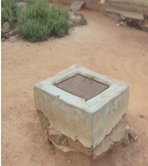
Figure 7: Non-functional covered well in Iju Source: Field survey, 2021
