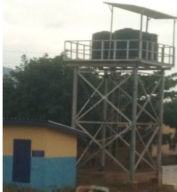
Figure 8: Solar powered borehole in Itaogbolu Source: Field survey, 2021
