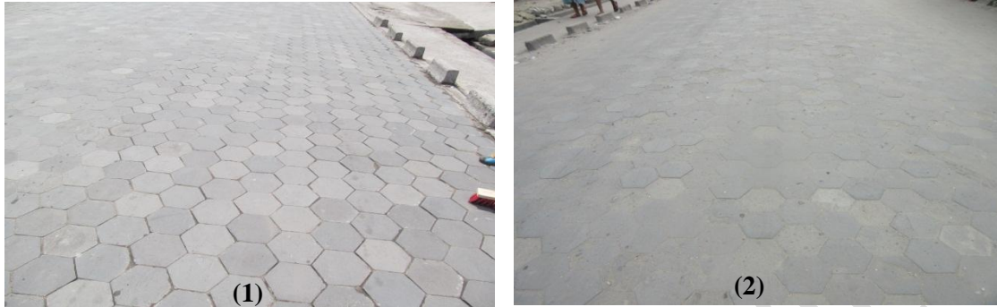
Figure 4. View of the paving stones at the start of installation (1) and after 8 years (2)
