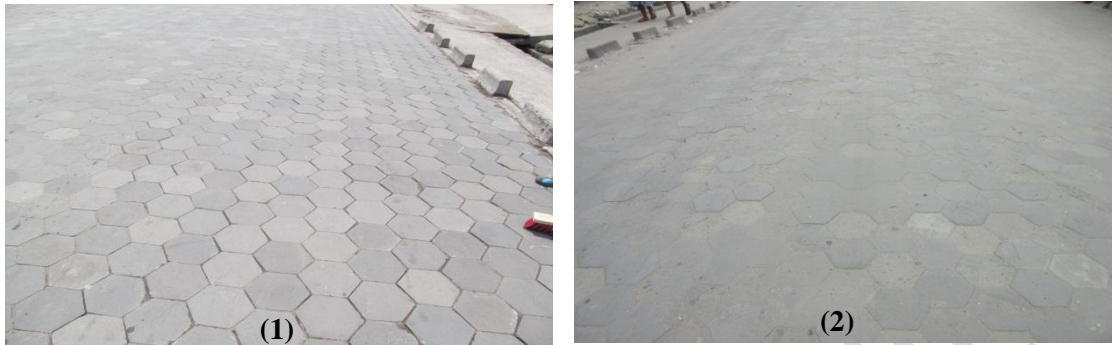
Figure 4. View of the paving stones at the start of installation (1) and after 8 years (2)
