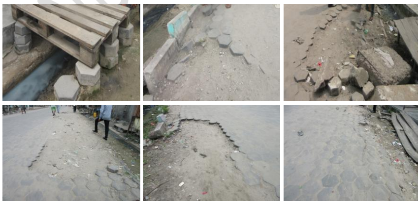
Figures 5. View of dilapidation of the framing edges
