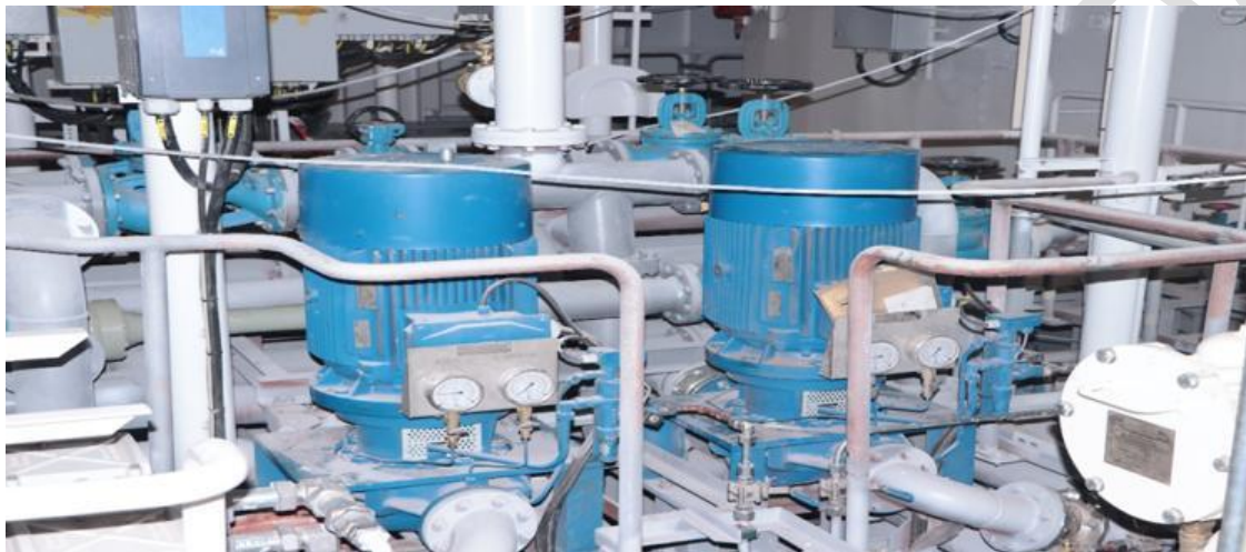
Fig-21 ballast motors
