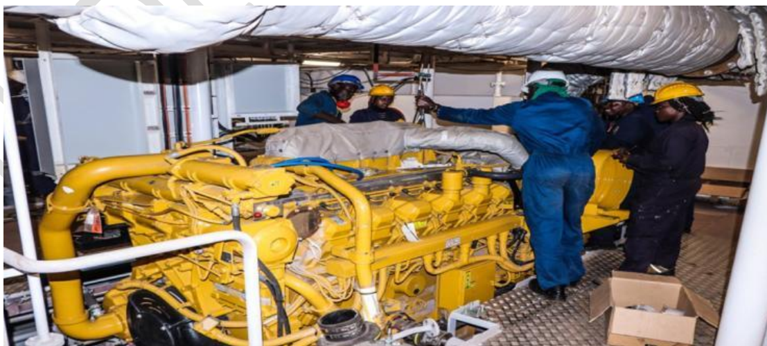
Fig-20 Main engines
