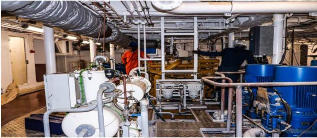
Fig-19 Piping system
