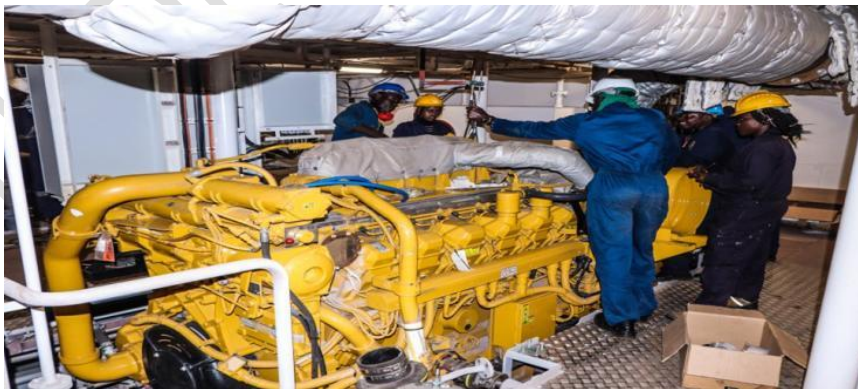
Fig-20 Main engines
