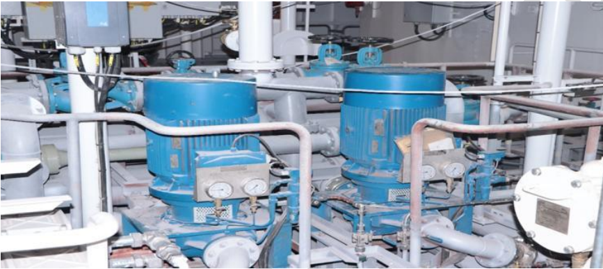
Fig-21 ballast motors
