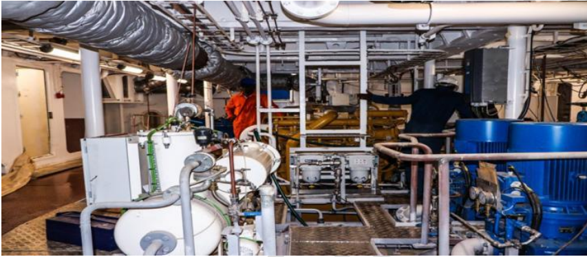
Fig-19 Piping system
