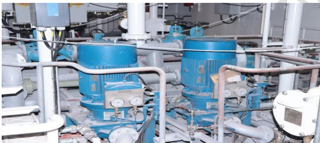
Fig-21 ballast motors
