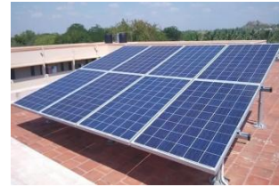
Figure 5. Solar Roof Top PV Panel system
