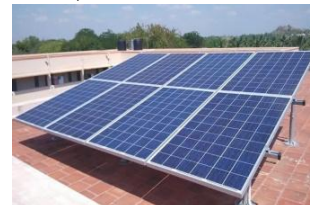
Figure 5. Solar Roof Top PV Panel system
