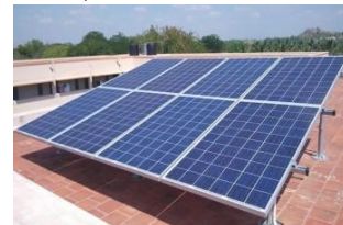
Figure 5. Solar Roof Top PV Panel system
