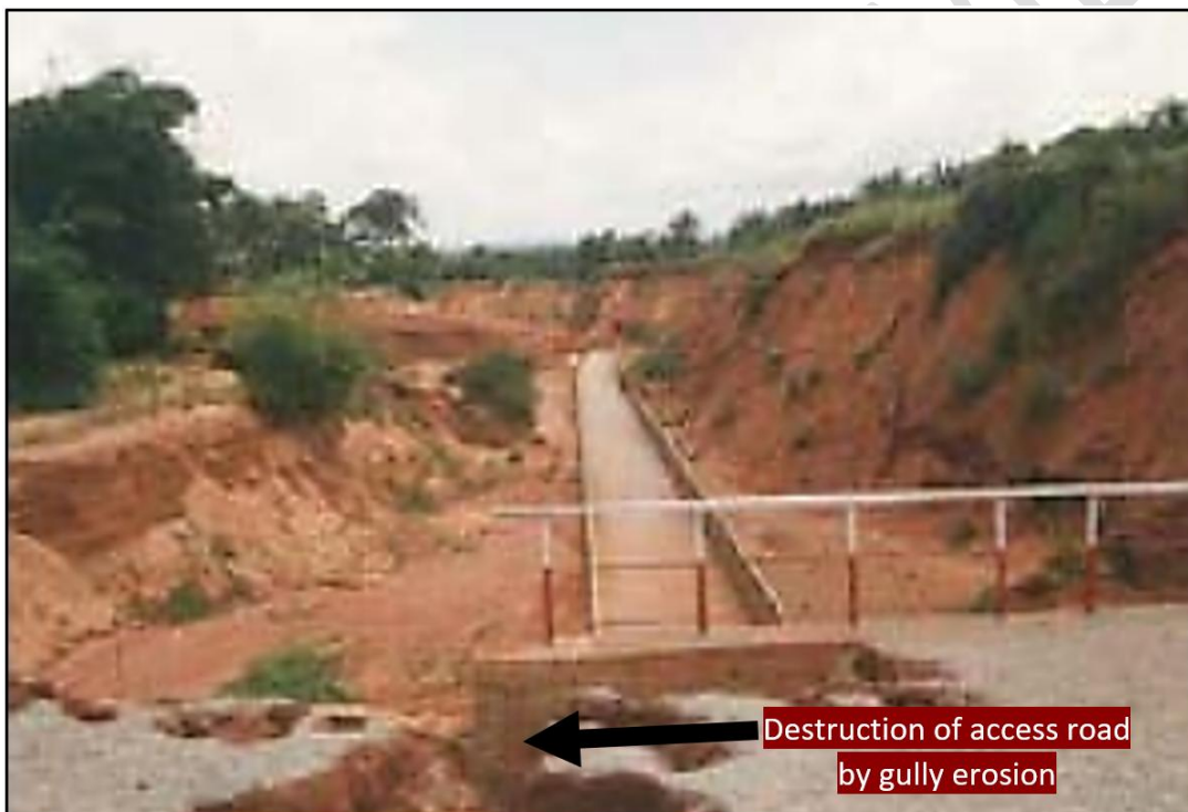
Fig 6: A Gully Site in Umuchiana, Aguata, showing the dissection of the access road [12]
