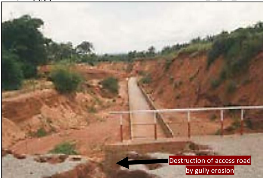
Fig 6: A Gully Site in Umuchiana, Aguata, showing the dissection of access road [12]
