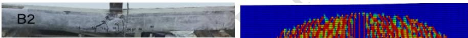
a) Cracking Patterns for Beam (B2) [EXP]. b) Cracking Patterns for Beam (B2) [FEM].
