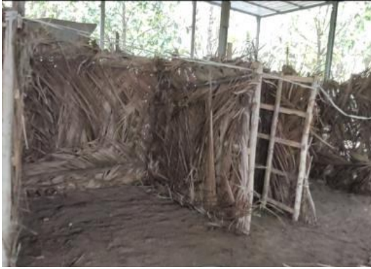
Pic. 4 : Support structure for erecting Novcom coir pith compost heap at Mandya, Karnataka.
