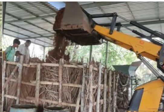
Pic. 8 : Transfer of cow dung slurry mixed Coir pith by JCB for erection of Novcom heap at model farm, Mandya, Karnataka.
