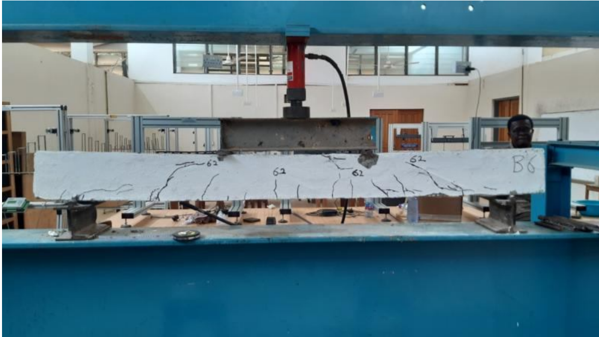
Figure 14: Beam 6 failure mode
