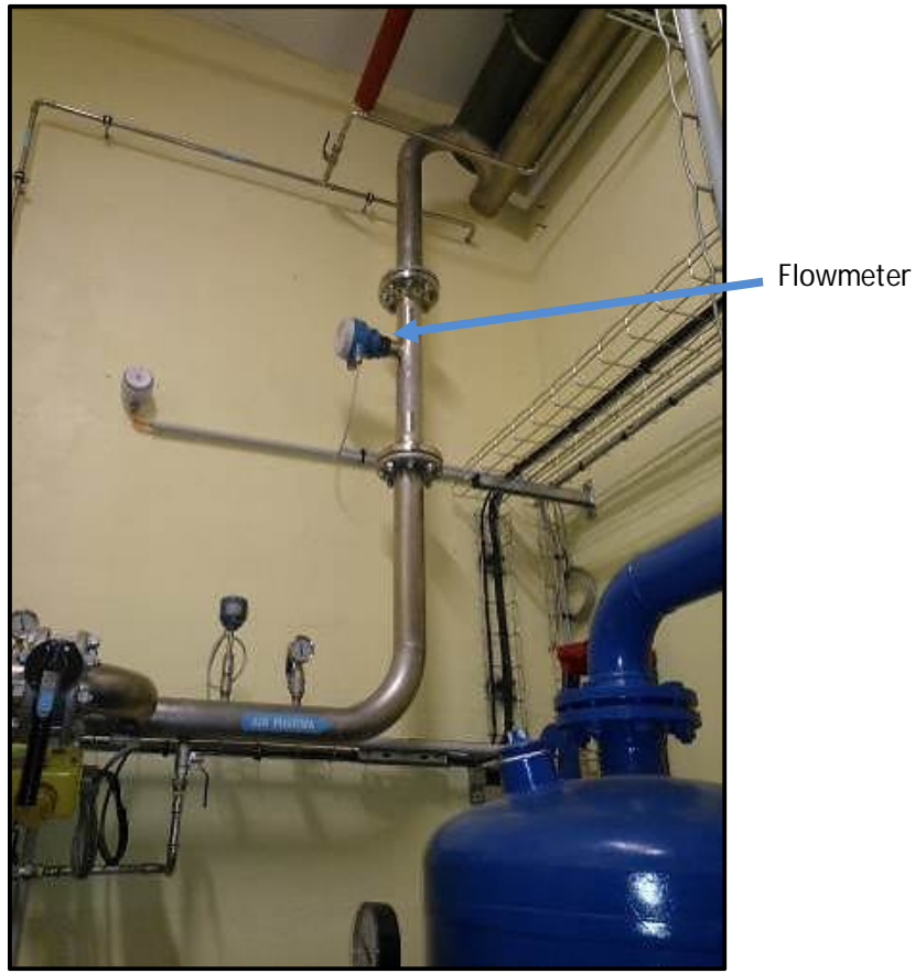
Figure 4: Compressed air flowmeter location
