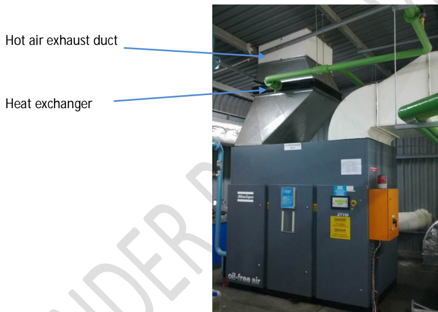
Figure 9: Example of heat recovery on a compressed air to produce hot water thanks to an exchanger
