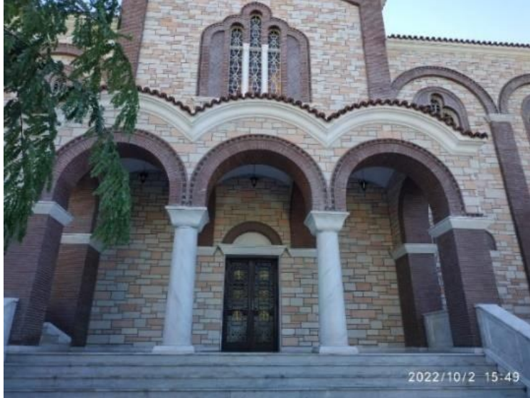
Figure 20. A Non-linear structure (Church) in a natural environment with few trees and without PnPlinear geometries → No Birds' nests found.
