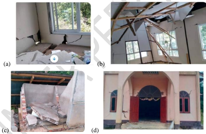
Fig.5. Mosaic of photos (a,b,c,d) show damages to the buildings in Kyaing Tong (Source-internet)
