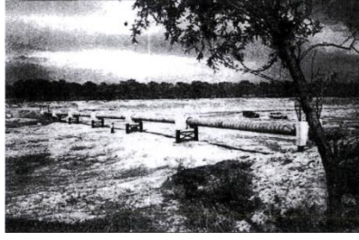
Figure 6 Severe exposure of an oil pipeline through a dike in the northeast (1997 situation)
