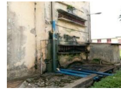
Plate 5. showing condition of Hostel Building, Cross River State University of Technology
