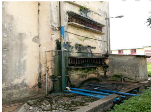
Plate 3: showing condition of Hostel Building, Cross River State University of Technology
