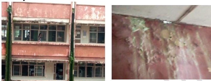
Plate 1: Showing condition of external/internal walls of university of Calabar library building.
