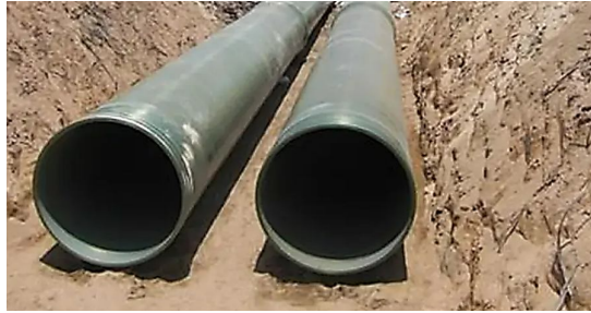
Fig.1. Hydroelectric power station pressure piping
