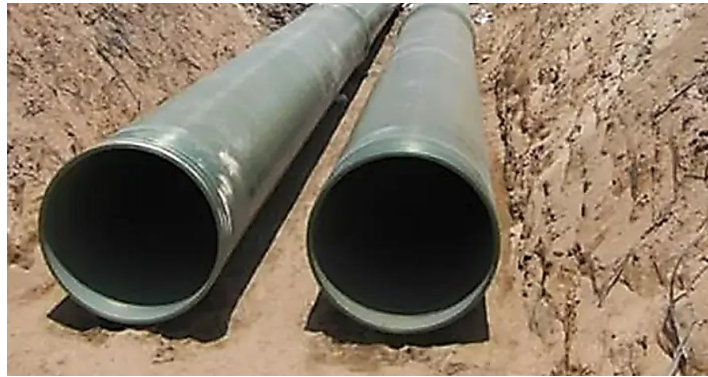
Fig.1. Hydroelectric power station pressure piping
